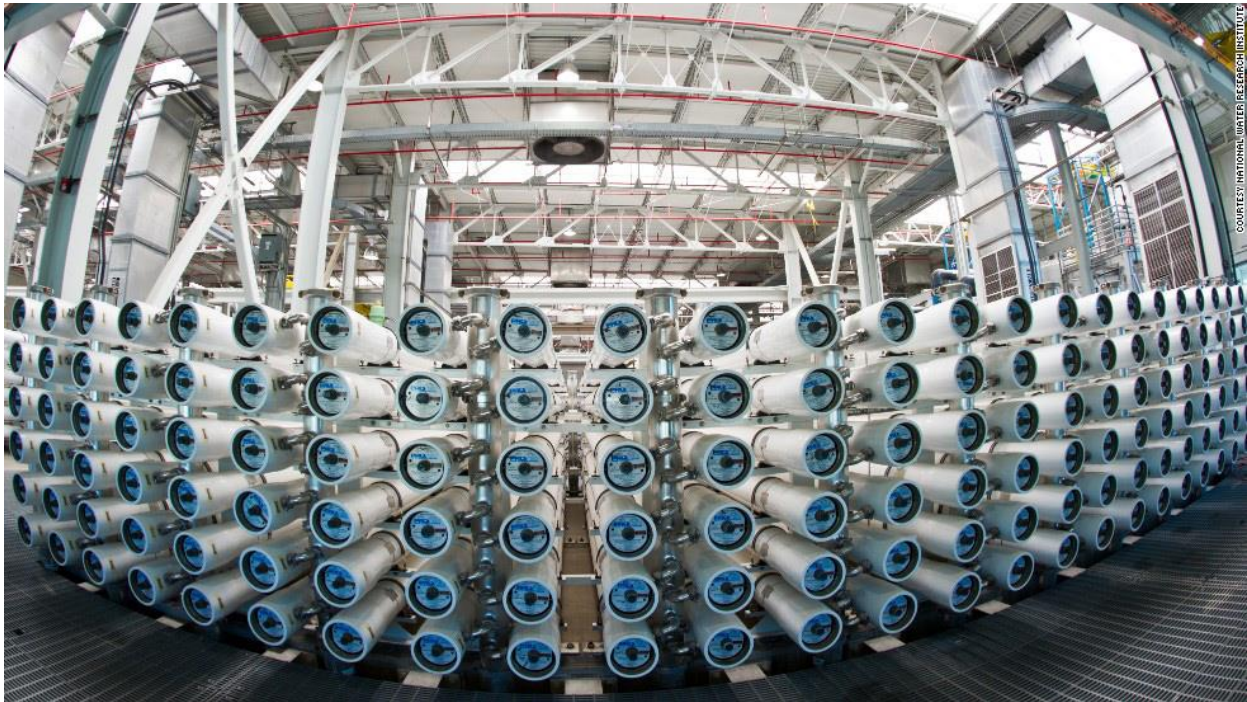
OCWD Reverse Osmosis Array, Fountain Valley, CA
